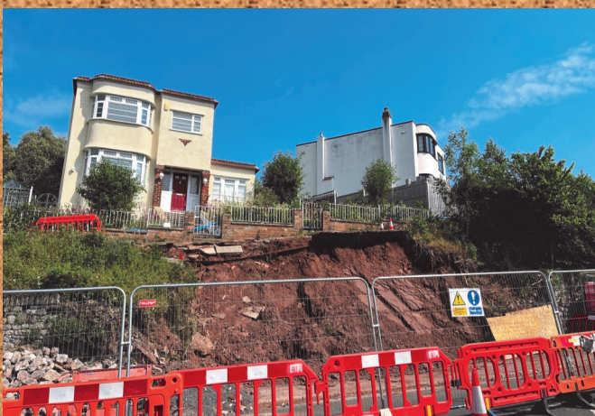
Our sympathies to these householders. A reminder to us all that steep slopes are increasingly apt to fail as the climate changes. (Photo by Judith Sheather)
